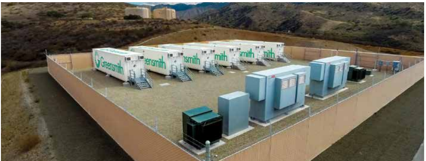
Figure 54: Greensmith battery storage system for distribution deferral in California
