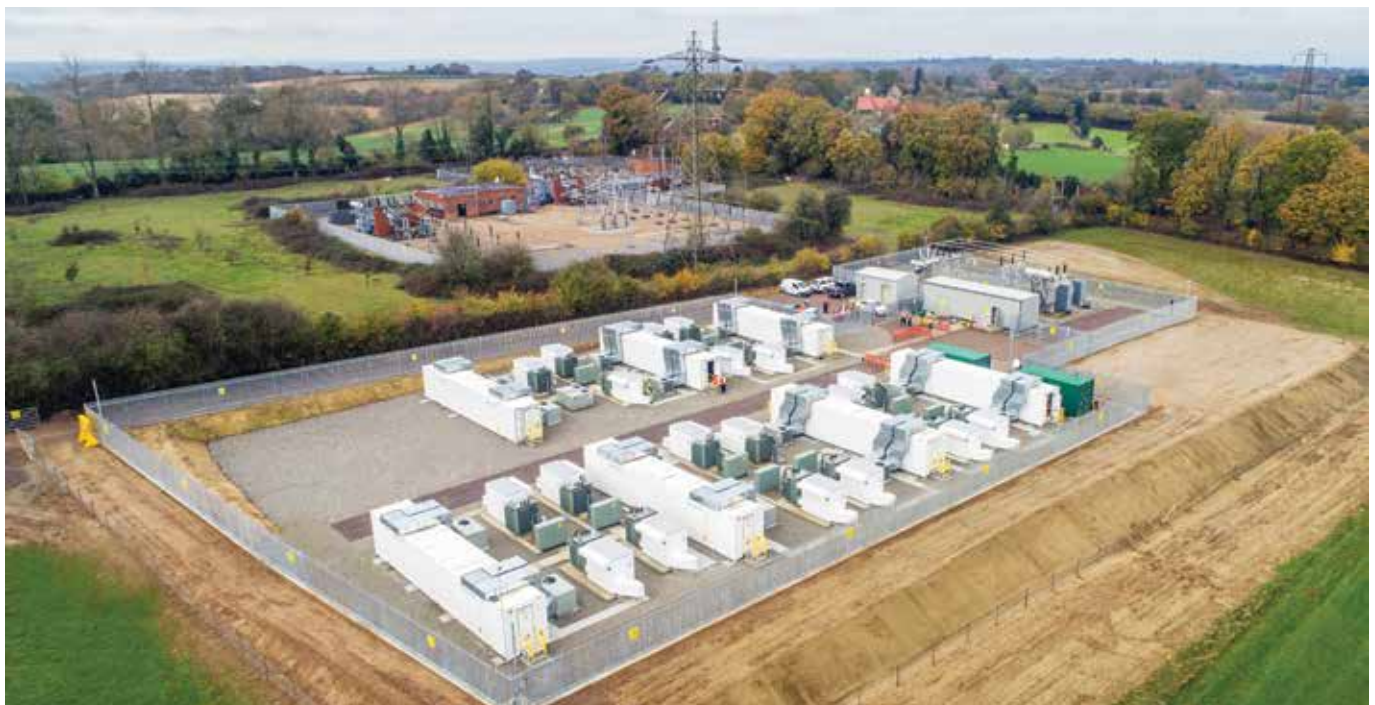
Figure 31: Low Carbon’s Glassenbury project
