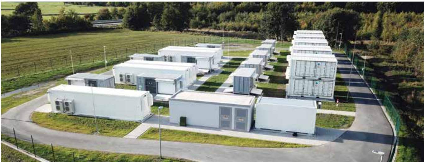
Figure 53: NaS batteries from NGK in Varel (Germany), similar to the ones in Campania region
