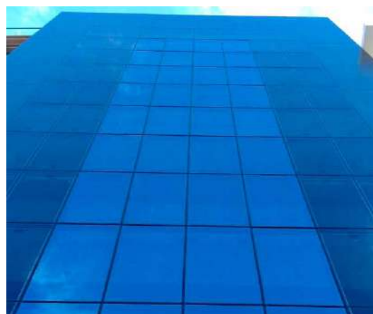
Fig. 4.2 a-Si BIPV glazed facade. Source: Onyx Solar.
